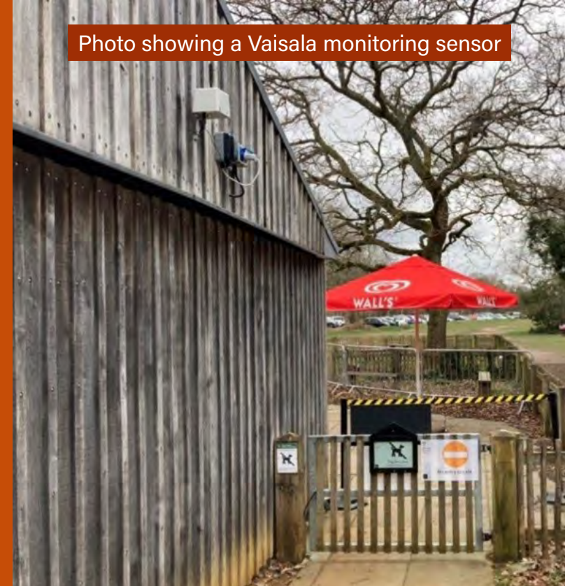
Photo showing a Praxis Cube monitoring sensor
